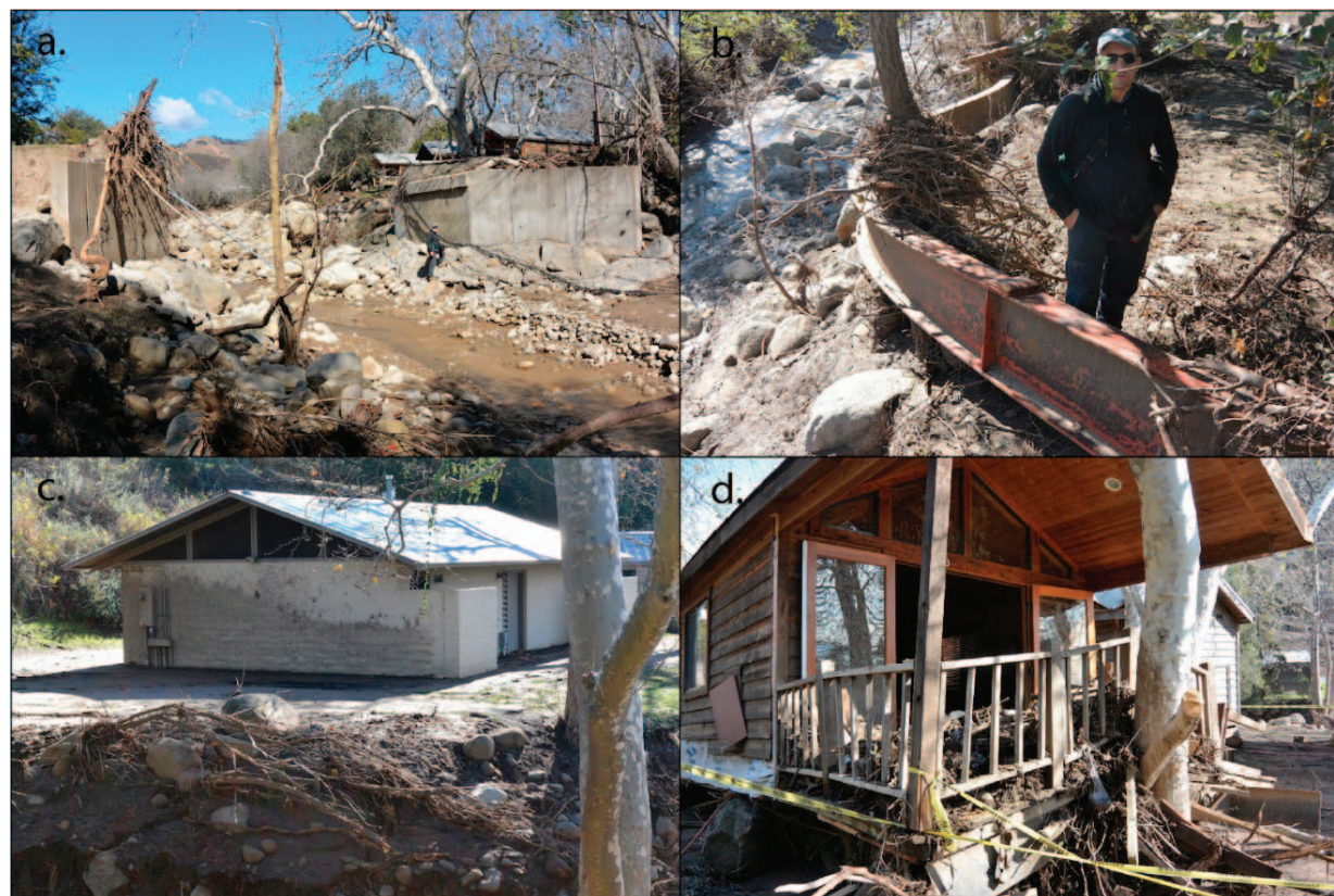
Figure 10. (a) Damage to the Mid-Canyon Bridge, supported on both sides of the creek by concrete abutments. (b) Twisted metal I-beams that supported the Mid-Canyon Bridge prior to the debris flow event. (c) Structure on the flood plain marked on its up-stream side by mud patinas to a height of up to 2.5 m. (d) Damaged cabins at the El Capitan Canyon Resort.
