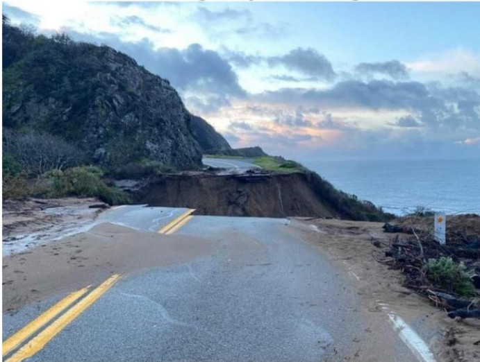
Landslide on Highway 1 near Big Sur, CA
